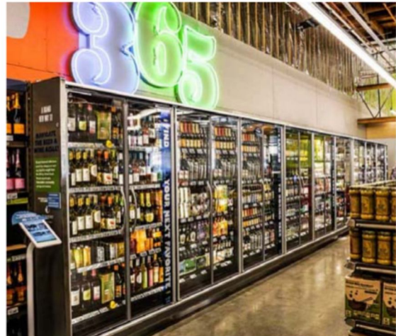
The Infinity 060 cooler doors installed at the new 365 by Wholefoods Market™ in Silver Lake, CA.
